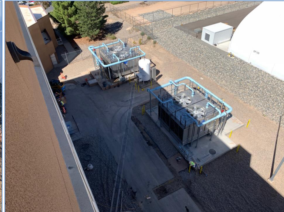
New cooling towers(1500-tons) installed.
