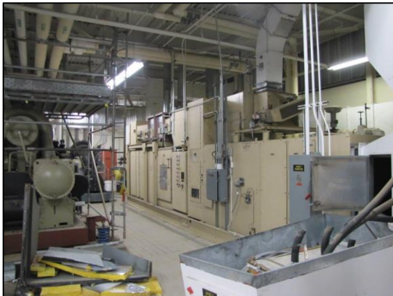
Existing RCHC-05 and ADE-01
